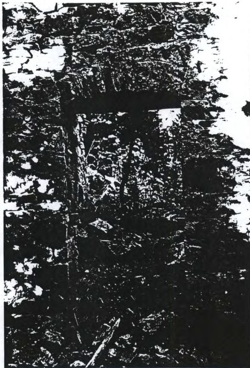
Figure 5. Christenot Mill (24MA1215) example of weakening of wall above unframed doorway, view looking west. (Roll:MBS/96-10, Frame: 7)
